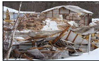
Roof Collapse in Guilford, ME 3/3/08 (Bangor Daily News)
